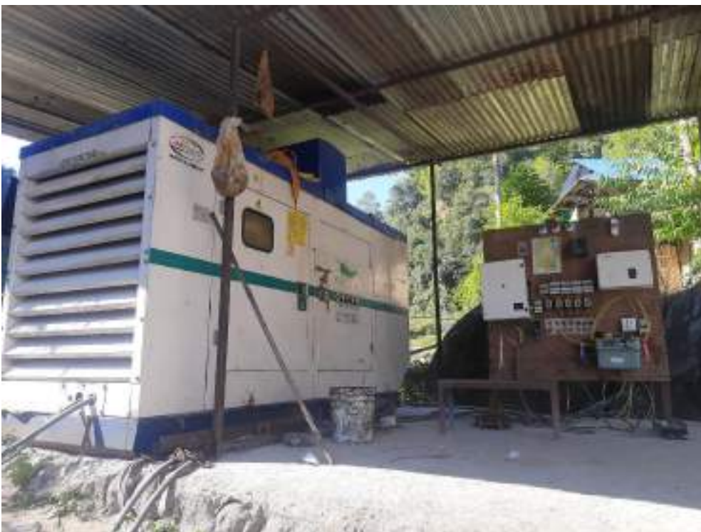
Figure 4-7: DG of 128 Kva used for crusher plant
